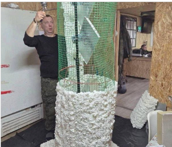
Foam Tree Stump Concealing a Communication Node, Colored and Shaped to Match Surrounding Trees. Source: serhii_flash
